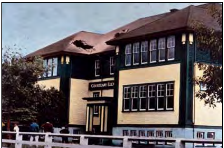
The 1946 Vancouver Island earthquake (M7.3) caused a chimney to fall through the roof at this school. New building codes in both Canada and the United States require much stronger structures, but thousands of schools and other buildings have not been updated to meet current codes. Photo: Natural Resources Canada (NRCan)
