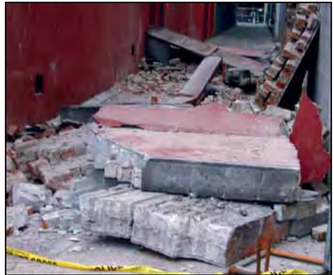
The last damaging earthquake in Cascadia was the M6.8 Nisqually event on February 28, 2001. This debris from a URM in Olympia fell in an alley and no one was hurt. Because it was a deep earthquake, the intensity of the shaking was less than it would have been in a similar-sized shallow earthquake. Photo: University of Washington Civil Engineering Department
