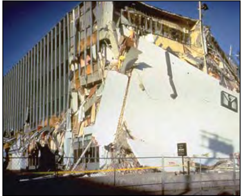
This building was of older, non-ductile, reinforced concrete-frame construction. End walls collapsed and separated from the main unit over the full height of the building. Photo: M. Celebi, USGS
