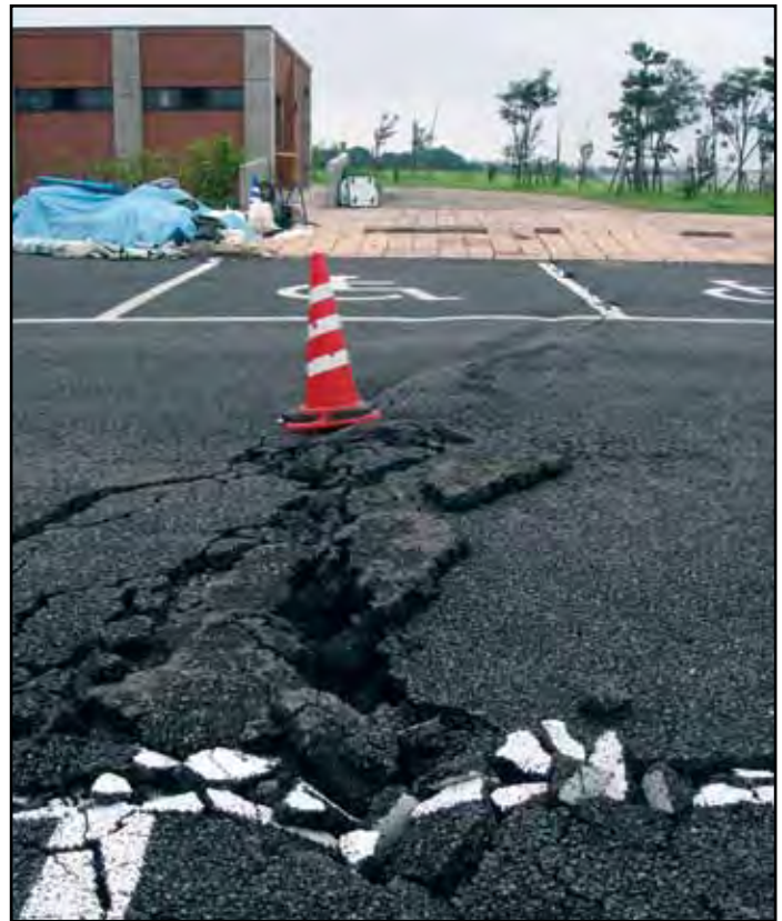
Lateral spreading and differential settling broke up this road and brick walkway. The same processes can severely damage buildings. Photo: Yumei Wang, DOGAMI
