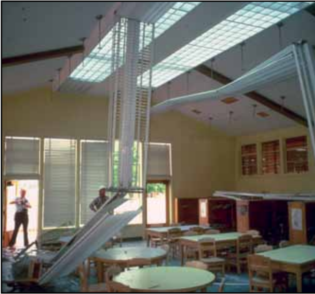
Failure of pendant light fixtures in this elementary school library could have caused injuries if the room had been occupied. Strengthening nonstructural elements in homes, schools, and offices can often be done easily and relatively inexpensively. Photo: EERI
