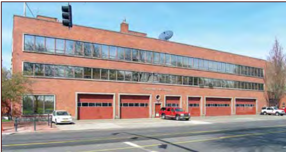
Built in 1952, Fire Station #1, is the largest in Portland. Its original concrete frame made it susceptible to serious damage in an earthquake. Strengthening work on the station, completed in 2009, included injecting cement into the soil beneath the building to prevent liquefaction and building settlement. It should now be in working order after an earthquake, serving downtown Portland. Photo Credit: Peck Smiley Ettlin Architects
