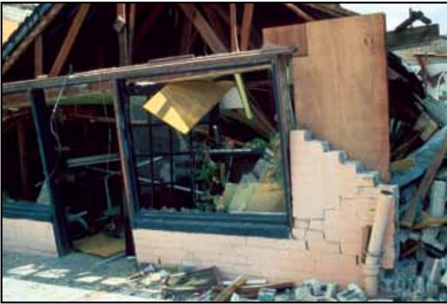
When brick, exterior walls fail, as in this store in Coalinga, they can injure people, block sidewalks and streets, or bring down utility lines. Photo: M. G. Hopper, United States Geological Survey (USGS)
